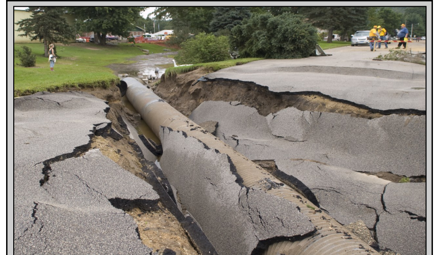
Drainage systems obstructed with trash or other debris can cause an increased risk of flooding since the floodwaters have no place to drain. The increased flooding caused by those obstructed drains can severely undermine the local roadway infrastructure structure, leading to potential health and safety hazards.
