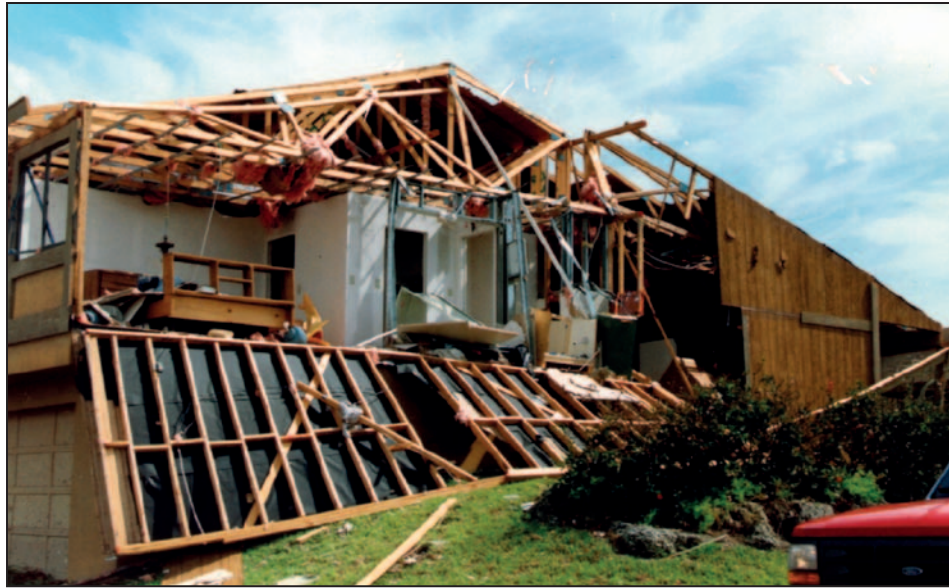
Figure 3-8. End-wall failure of typical first-floor masonry/ second-floor wood-frame building in Dade County, FL (Hurricane Andrew, 1992)
