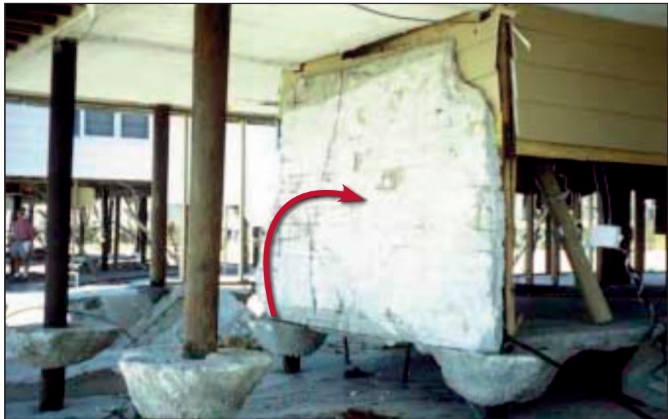
Figure 3-26. Concrete slab-on-grade flipped up by wave action came to rest against two foundation members, generating large unanticipated loads on the building foundation (Topsail Island, NC, Hurricane Fran, 1996)
